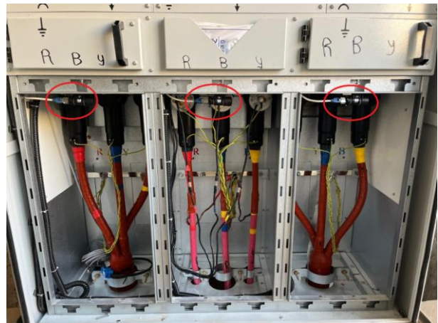
Figure 2 – Images of sensor installation at trial sites
