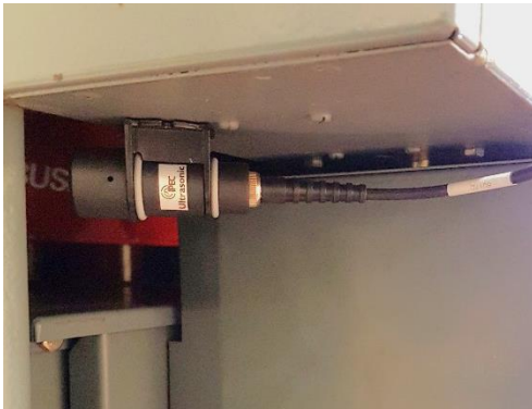
Figure 2. A photo of an AA sensor installed on VMX AIS with the transducer pointing through a large gap at the breaker spouts.
