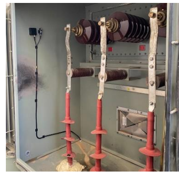
Figure 6. A photo of a transformer termination enclosure with a UHF sensor and an AA sensor mounted internally.
