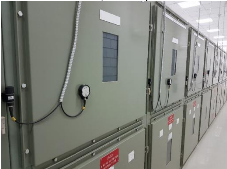
Figure 1. A photo of transient earth voltage (TEV) sensors installed on metallic switchgear panels and AA sensors
