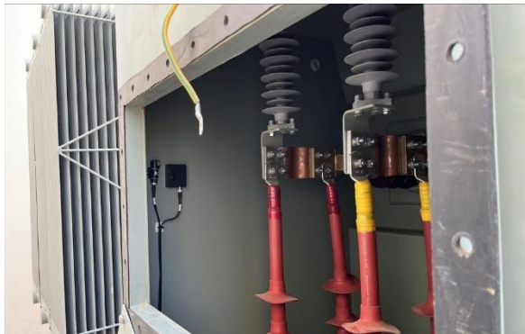
Ultrasonic and UHF sensor installed on Transformer
