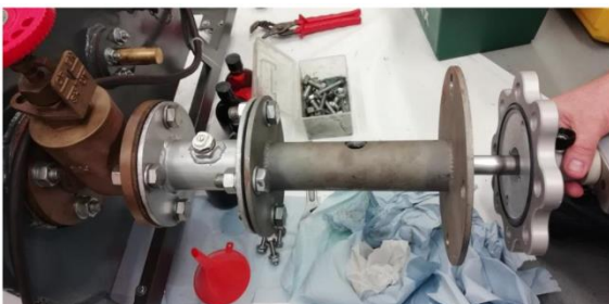
Drain valve sensor installed on Transformer
